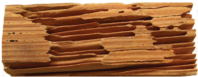
Figure 14–13. Shelter or “mud” tubes (top), subterranean termite foragers (middle), and pine wood showing typical termite-damage (bottom).
