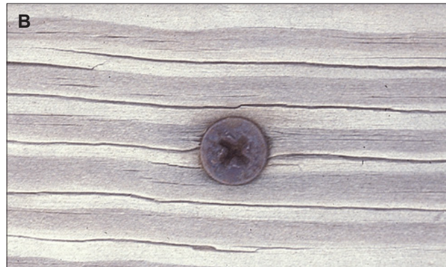
Figure 16–27. (A) Iron stain on newly installed cedar siding. Poor quality galvanized nails corrode easily and, like uncoated steel nails, usually cause unsightly staining of the wood. (B) Pine, on the other hand, does not contain appreciable tannins, so iron stain is not an issue even with rusty fasteners.
