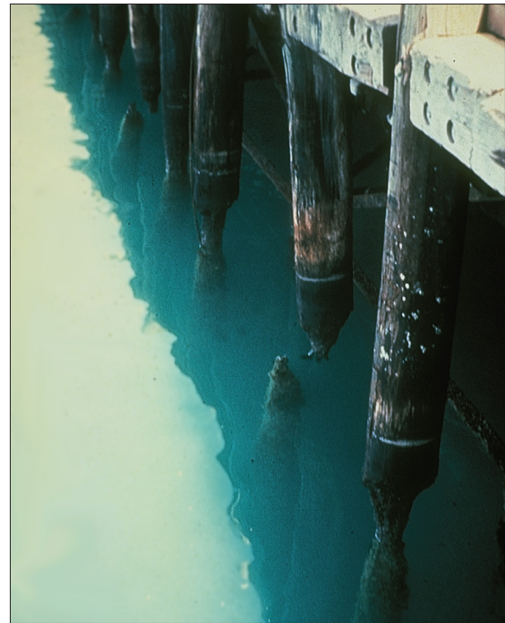
Figure 14–15. Limnoria damage to piling.
