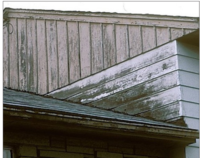
Figure 16-15. The siding came too close to the roof, absorbed water from the roof, and rotted.
