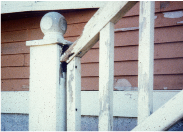
Figure 16-13. Decay and paint failure in wood railing that trapped water. Problems could have been minimized by priming all surfaces before assembly to prevent water entering the wood.
